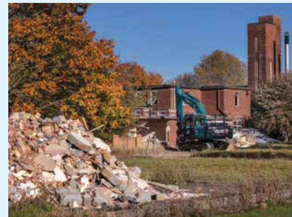
Demolition of Building 63 – built in 1940 and refurbished in 1990 – and used as offices and store/armoury
